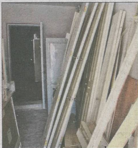
DAMAGE: When the drywall was taken out, blackened pipes were revealed.
